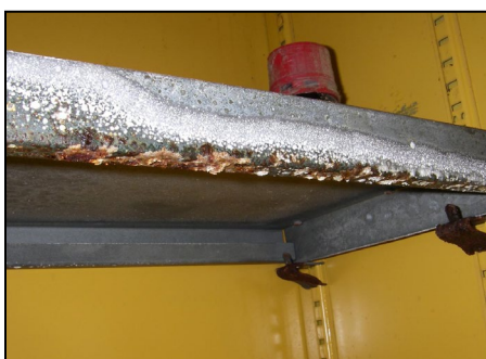
Rusted shelf supports
