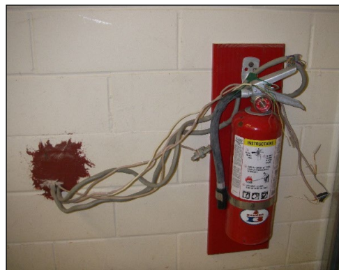
Blocked fire extinguisher
