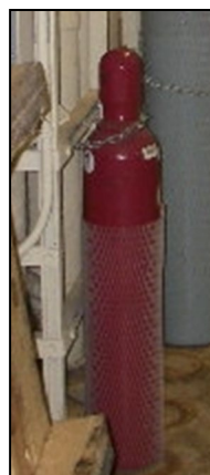
Unacceptable method of securing a gas cylinder
