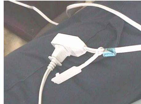
Electrical cords daisy-chained
