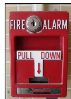
Fire alarm pull station
