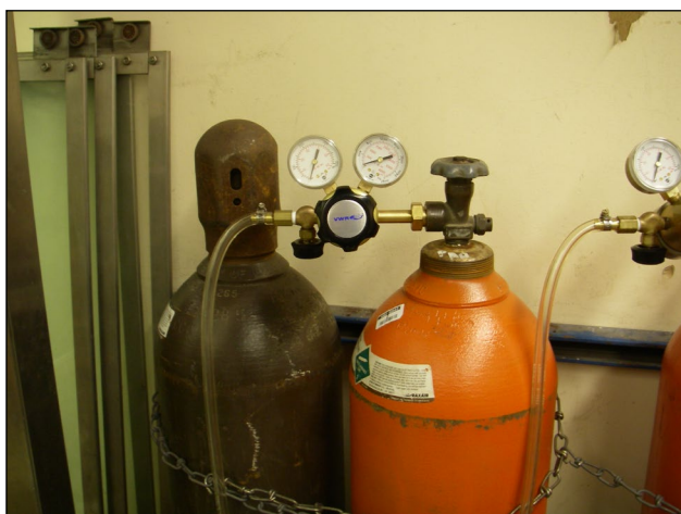
Properly attached regulator and safety cap (left) adjacent to operating cylinder with regulator attached
