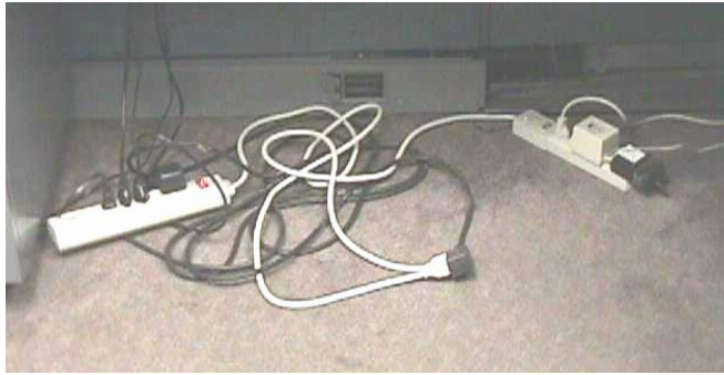
Overloaded multi-plug strip
